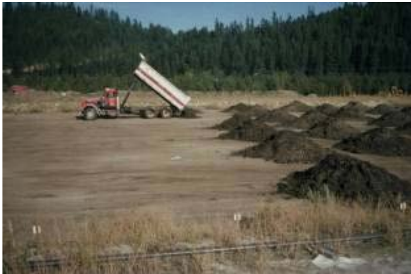
Contaminated soil being placed in a treatment cell at the Libby Superfund Site
