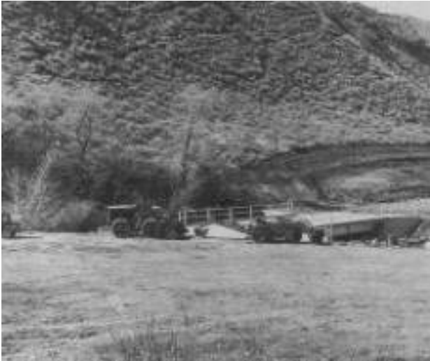
First step in the construction of the UWRL was the bridge across the river
