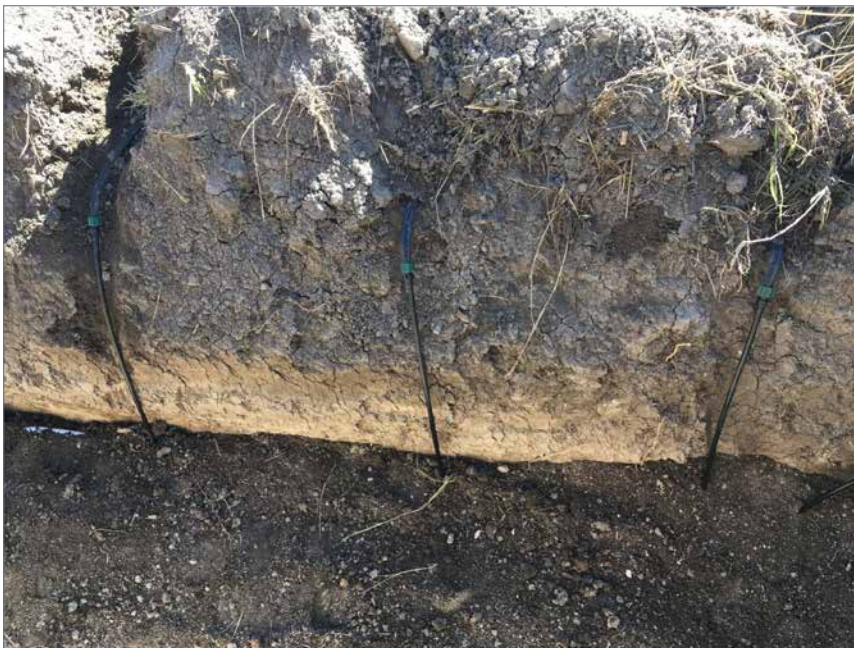
Figure 1: Subsurface drip irrigation tubing during installation. The tubing is fed from a mainline, which is partially buried in the foreground of the photo.
