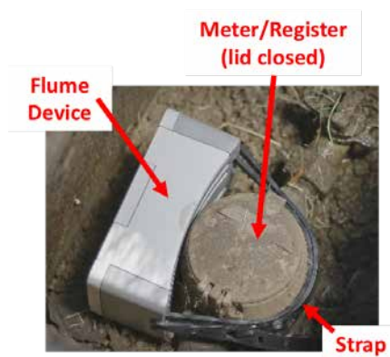
Figure 1: Flume, Inc. Smart Home Water Monitoring device (grey) strapped around a water meter.
