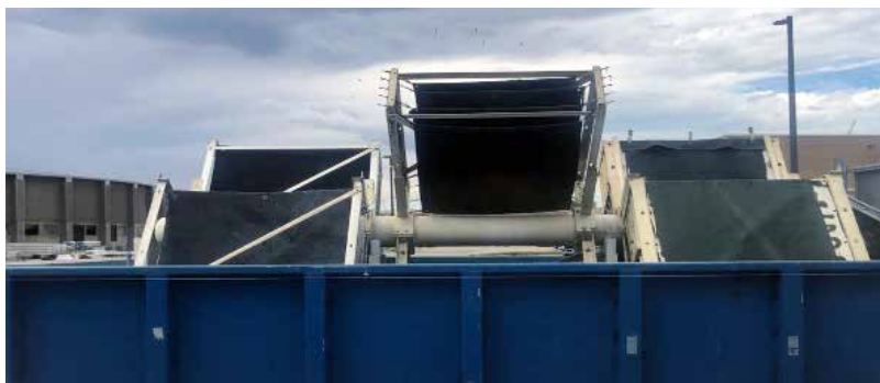
Figure 1: Algae biofilm reactor (RABR) at the Central Valley Water Reclamation Facility. Algae grows as a biofilm on the surface of 100% recycled plastic shelves and is harvested using mechanical scraping with a squeegee.
