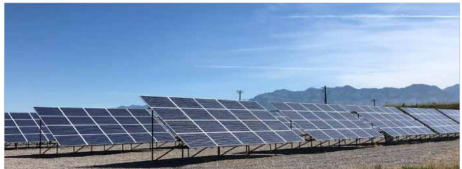
Figure 1: Community solar array installed adjacent to the Logan City Wastewater Treatment Lagoons
