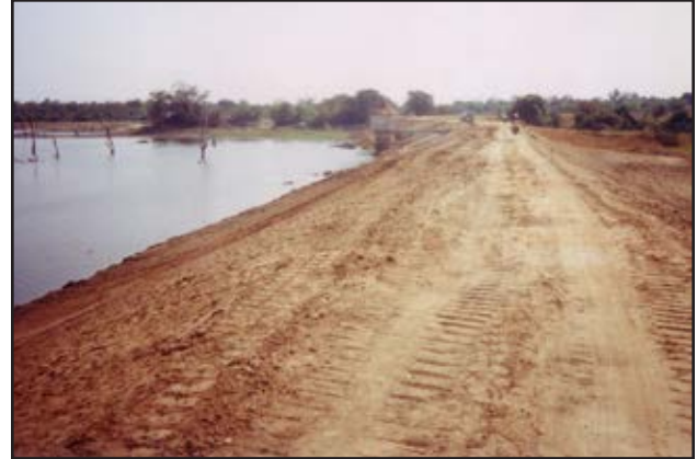
Upgrade work (embankment and spillway) on a "tank", a small reservoir used to store monsoon season rainfall for later use for irrigation. This tank was originally built between 1,000 and 2,000 years ago and had not been used for more than 800 years. The design of the modern irrigation and drainage systems brought these ancient structures back into use (Mahaweli River Basin, Sri Lanka)
